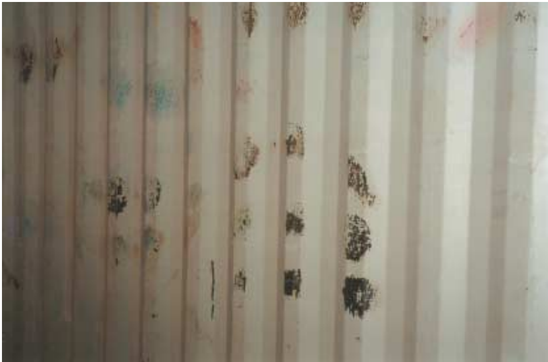
Large areas of paint failure and powdery rust. Requires localised de-rusting and painting.
