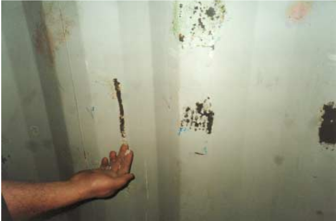
Loose and blistering paintwork. Requires localised treatment and repainting.
